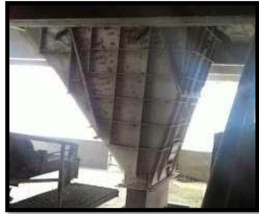
After up-gradation (Static Separator)
