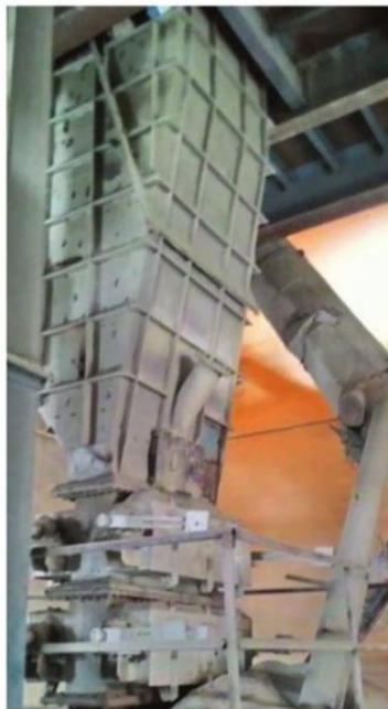
A static separator with an air volume of 165,000m 3 /h was installed
