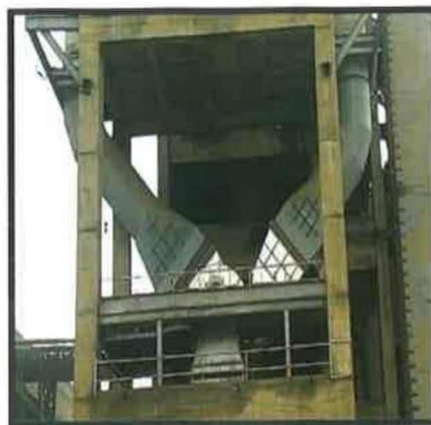
Circulating air fan for VRPM Circuit
